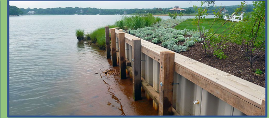
Bayside Bulkhead Construction – First Coastal. (2016, January 1). First Coastal. Retrieved January 25, 2025, from https://firstcoastal.com/bayside-bulkhead-construction/
